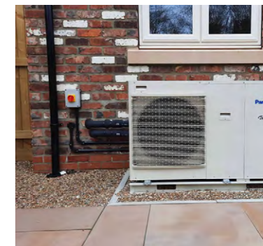
ref.14: Image showing Air Source Heat Pumps
